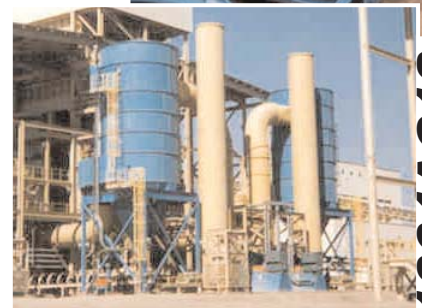
Two 1064AC12 attached to the transfer tower handles 40 tons of dust per day.
